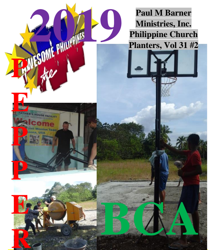
Arizona & Colorado work teams pour cement to build a basketball court at BCA's FHF orphanage.
