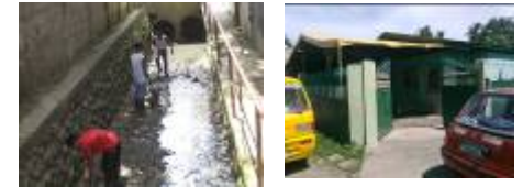
ONGOING PROJECTS: EMPTYING THE CANAL & FILLING OUR FHF HOME FOR STREET KIDS.
